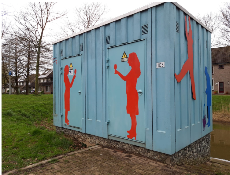
Figure 2: Secondary substation at De Randweg in Arnhem [Van Osch, 2021]
